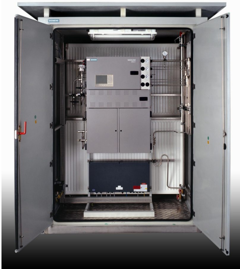
Water Cooled Gas Chromatograph for a Gas Plant in the Gulf area
