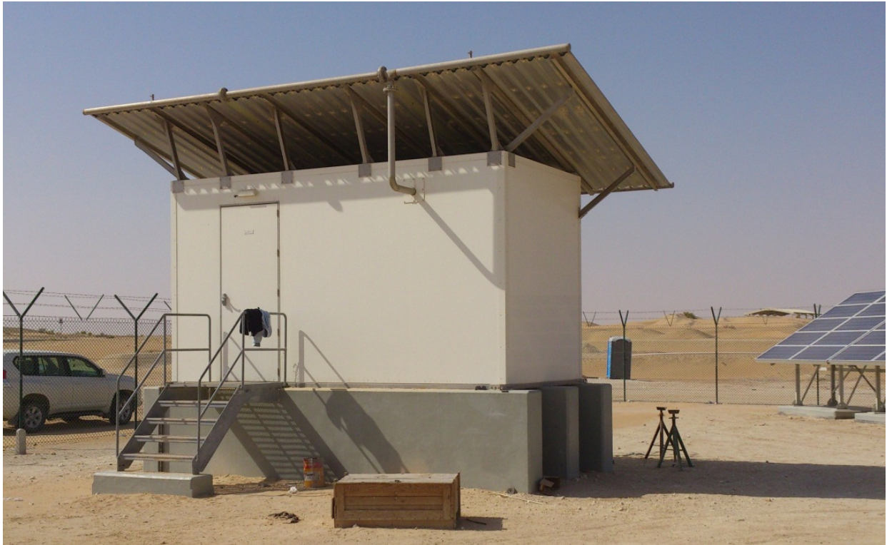
PCS Shelter for ADCO SAS project in the UAE/Sahil and Shah
