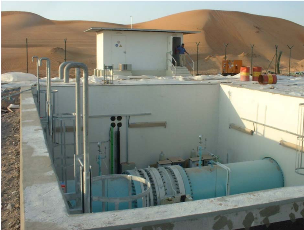
SCADA Shelter for a drinking water pipeline in the UAE/Fujairha
